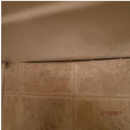
Seal Base of Tubs Where Meet Floors
