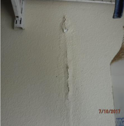
Damage in Garage
