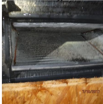
Evap. Coil Lacking Maintenance
