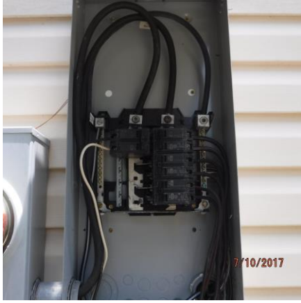
Main Panel in Good Order
