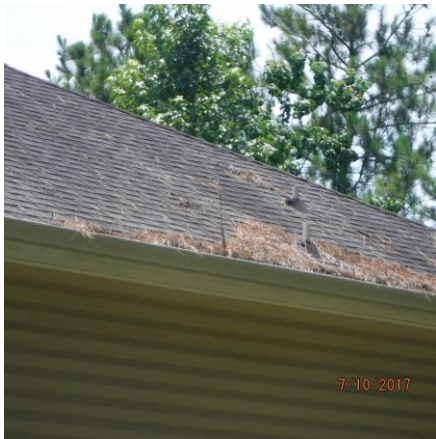
Debris on Roof – Typical
