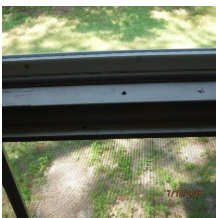
Window Hardware is Missing
