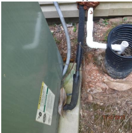
A/C Piping Insulation Damaged
