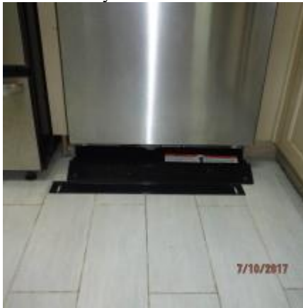
Base Plate Loose on Dishwasher
