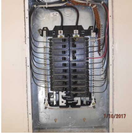
Auxiliary Panel in Good Order
