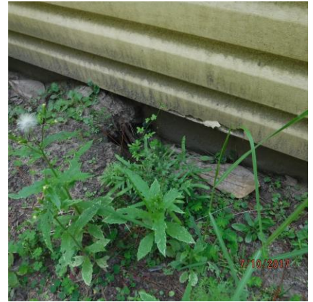
Erosion from Roof Discharge
