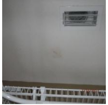
Ceiling Stains in Master Bed Room
